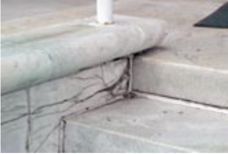
Due to harsh weather, marble is seen eroding from the steps at the front of the Butler historic facade.
